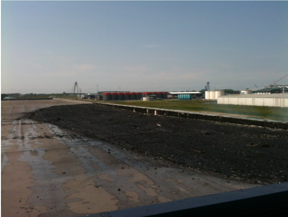
Figure 15 Overview of the damage to the roof (Source: Kampen fire department)
