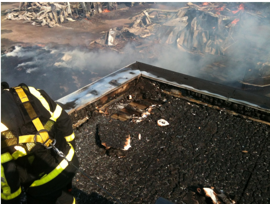
Figure 16 Damage to the roof of the Asia building (Source: Kampen fire department)
